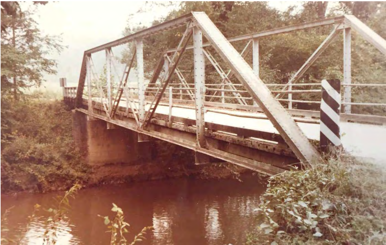
Bridge No. 95 (MC 125), SR 1161 over Catawba River [Photo from HPO Survey Files]
